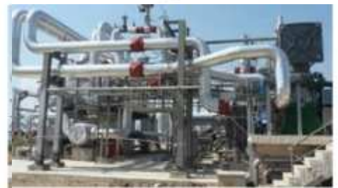
The Akça geothermal plant
