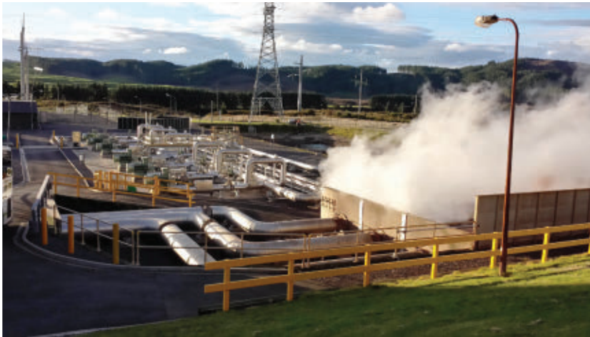
A geothermal plant in the Taupo, New Zealand area. Credit: Chris Webb.
