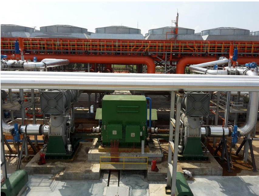
Karkey Geothermal Plant in Turkey (Source: Courtesy of EXERGY)
