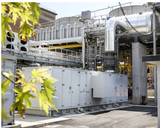
An Exergy ORC WHR cement plant, Italy, 2020.
